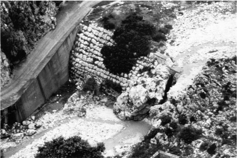
Fig. 220. Kandila, Glosses, Castle and 'Byzantine Nerotrivio'. View of the dam and Byzantine building from the Castle (courtesy of J. Knauss).
